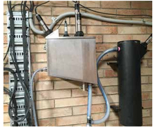
Final drinking water quality monitoring system using Xylem's pH, free chlorine, turbidity and conductivity sensors
