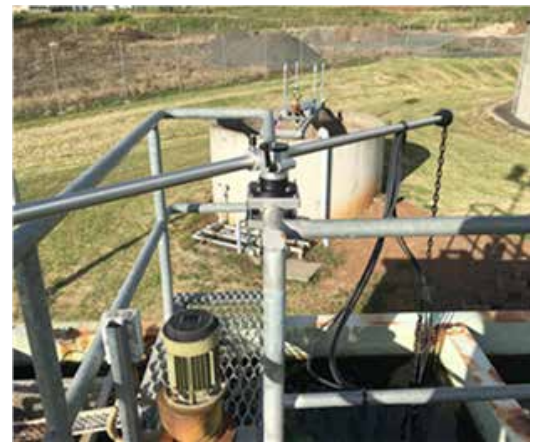
Raw water quality monitoring - using pH, turbidity and conductivity sensors suspended directly in the clarifier using a 3-sensor holder and swing mounted assembly on the handrail.
